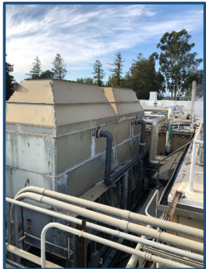
Cooling Tower Poor condition
