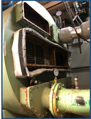
Abs. Chiller Over 30 yrs old
