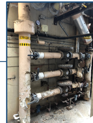
Steam Piping Needs renewal within 10 yrs
